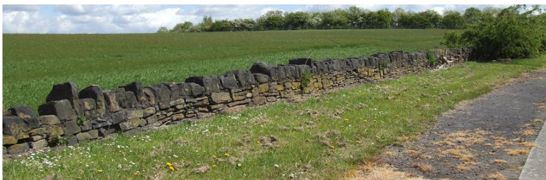
The old boundary wall across the road from the Cross Keys shows signs of great age in places.
